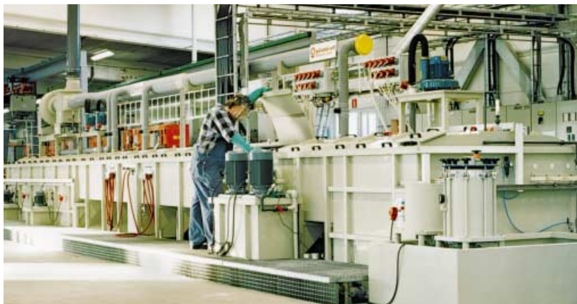
A new plant for nickel coating of spring wire was placed in operation at Gusab Stainless in Mjölby, Sweden.
