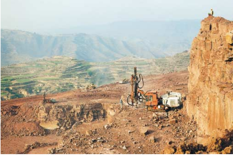
One of the world's largest civil-engineering projects is under way along the Huang Ho River in China. The hydro-power project will involve excavation of 30 million m 3 of rock, mainly with equipment from Tamrock and Sandvik.
