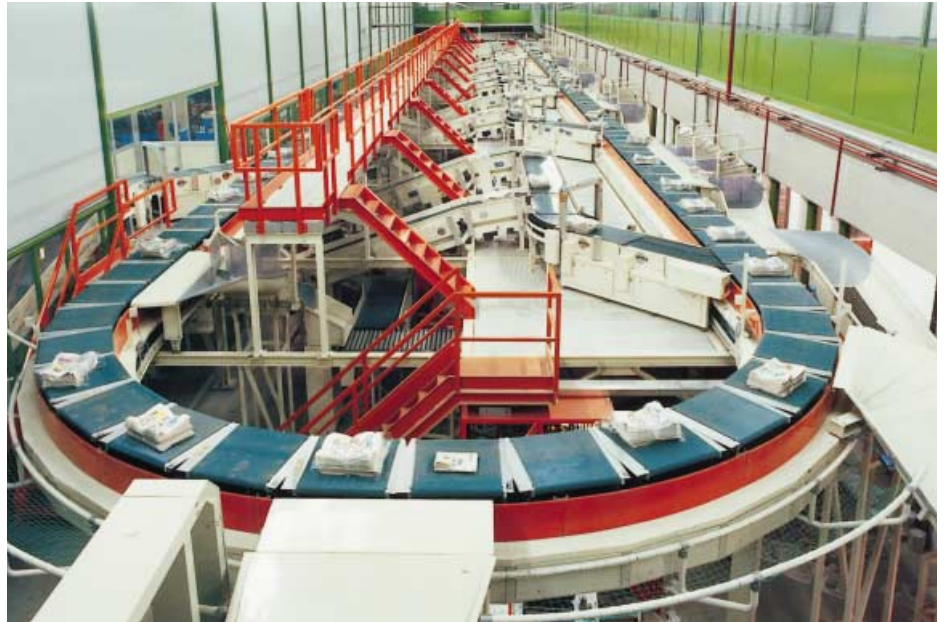
CML's SBIR sorting system for newspaper distribution is used by La Stampa, one of Italy's largest dailies.
