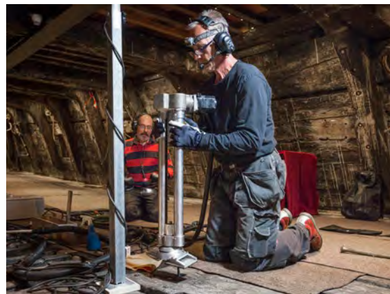
Sandvik has replaced 4,000 rusty bolts on the 17th century Vasa war ship at the Vasa museum in Sweden.
